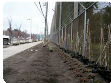
Swale section containing reactive filter media
