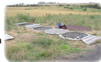
Figure 2. Treatment tanks at Toxic treatment Facility
